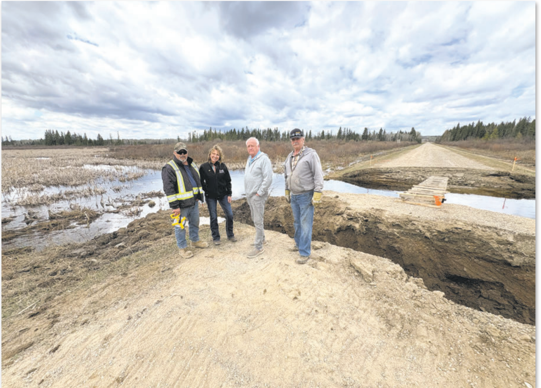
A 36-foot wash out on the main road in the Mayview area poses a large challenge for the R.M. of Shellbrook. Pictured: R.M. Foreman Todd Lande, Reeve Christine Strube, Agriculture Minister David Marit, and contractor Gary Sjogren tour the washout.
